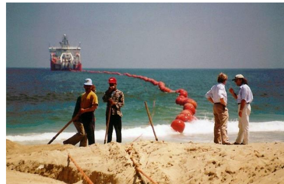
Fig. 10: Positioning the cable before digging, with the cable laying ship in the distance (© Sergio 77)
