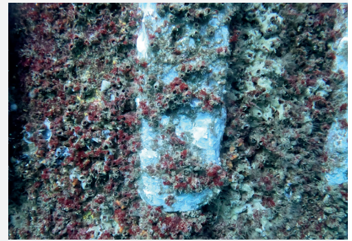
Biofouling developing on a galvanic anode Credit: ©FEM
