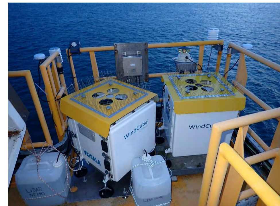
Two coupled-lidar profilers installed on the Fécamp met. mast
