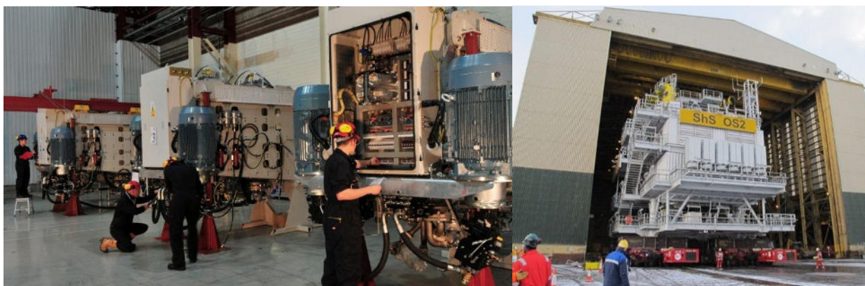
Figure 2.2.4-8: Pelamis engineers assembling motor generator sets (on the left), offshore substation leaving manufacturing facility (on the right).
